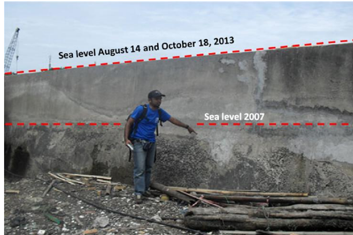
Figure 7: Subsidence along Jakarta waterfront
